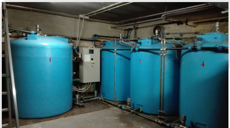
WDMS NT-VK example (decay tanks and PLC board)
